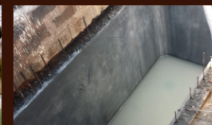
Sump Water Draping System
